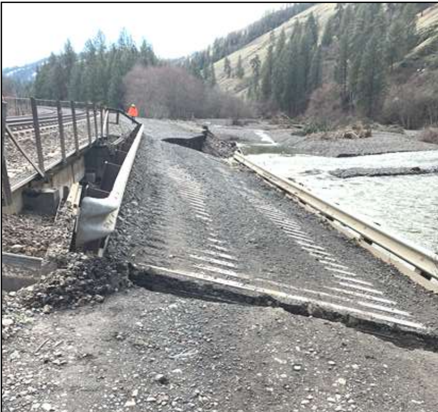
Damage to essential infrastructure from flooding, like to this railroad access bridge increases disaster recovery costs. Tribal Nations and local governments can reduce future costs by considering climate projections in current program and infrastructure development.
