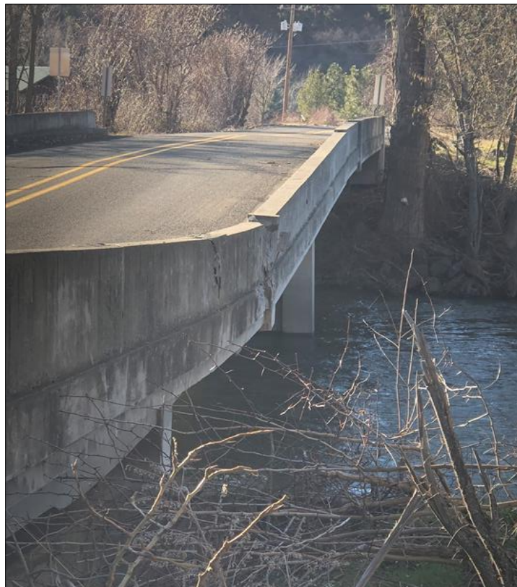
Thornhollow Bridge on the Umatilla Indian Reservation was damaged by the February 2020 flooding. Note the buckled concrete in the bridge center.
