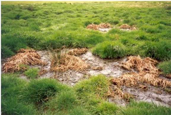
Sewage surfacing on the ground, like in the picture above, is a sign of a failing septic system.
