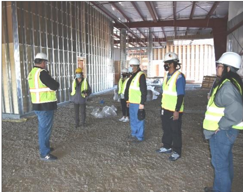
CTUIR Board of Trustees and other representatives tour the DCFS Tutuilla Food Sovereignty Center under construction in 2021. New infrastructure developed to withstand historic conditions will be unprepared for future conditions with greater stress on systems.
