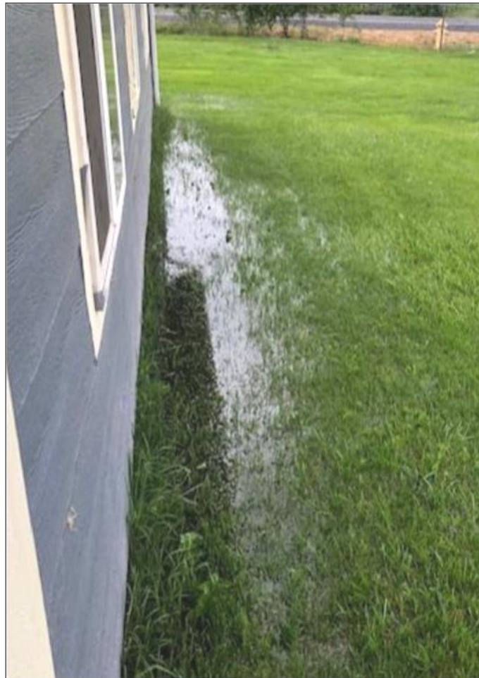
Mission area housing has experienced inundation from rising groundwaters, also known as a spring, which is located in the floodplain of nearby Mission Creek.
