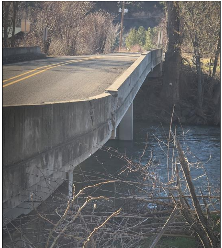
Thornhollow Bridge on the Umatilla Indian Reservation was damaged by the February 2020 flooding. Note the buckled concrete in the bridge center.
