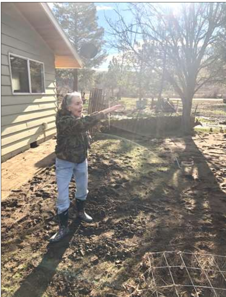
Judy Beers, a UIR resident, surveys damage to her home and property from the Feb 2020 flood. Inundated homes are at a greater risk for developing mold issues.
