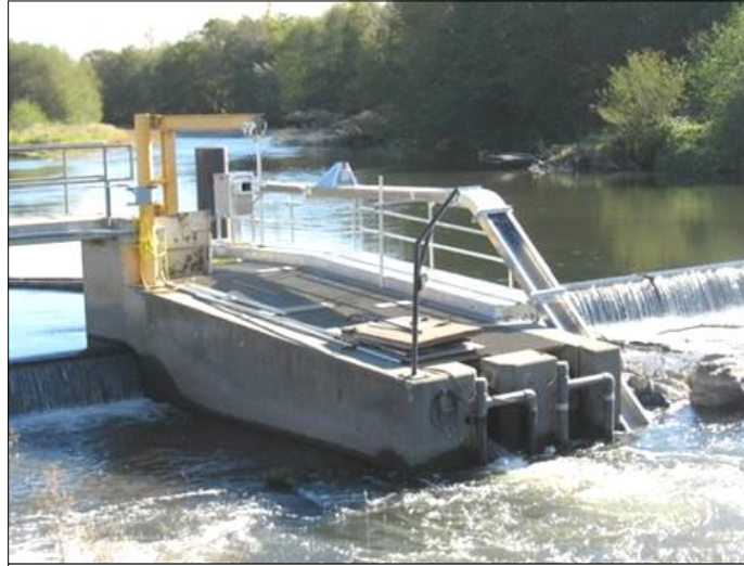
Fisheries support infrastructure like hatcheries, rearing ponds, and fish ladders could be excellent locations to co-locate microhydro generating opportunities due to their essential proximity to stream flows.
