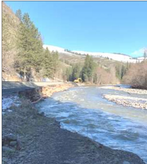
River-adjacent infrastructure, such as the Union Pacific Railroad line along Meacham Creek (pictured left), is threatened by flooding and also impedes floodplain reconnection.
