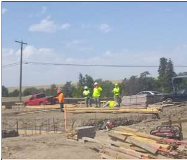
Construction workers take a break from work on the new Nixyaawii apartment buildings under extreme heat which will become more frequent.
