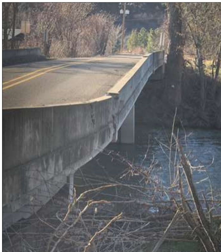
Thornhollow Bridge on the Umatilla Indian Reservation was damaged by the February 2020 flooding. Note the buckled concrete in the bridge center.
