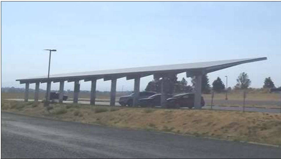
Passive energy strategies like PV shading for parking facilities. This one at TCI (pictured) provides electricity generation and reduces heat island impacts.
