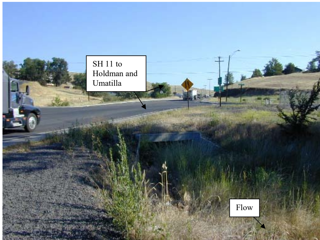
Photo No. 44: View looks north at Nelson Creek concrete box culvert under SH 37.
