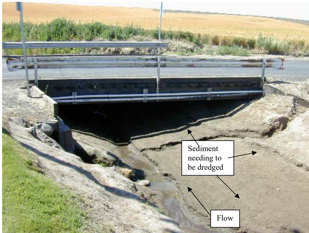
Photo No. 33: View looks south at upstream side of Greasewood Creek bridge at west edge of town.
