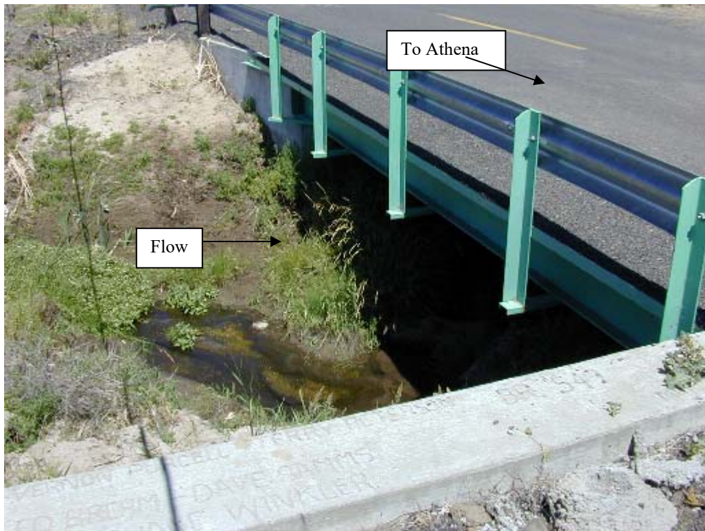
Photo No. 9: View looks at upstream face of bridge over Waterman Creek/Gulch north of town.
