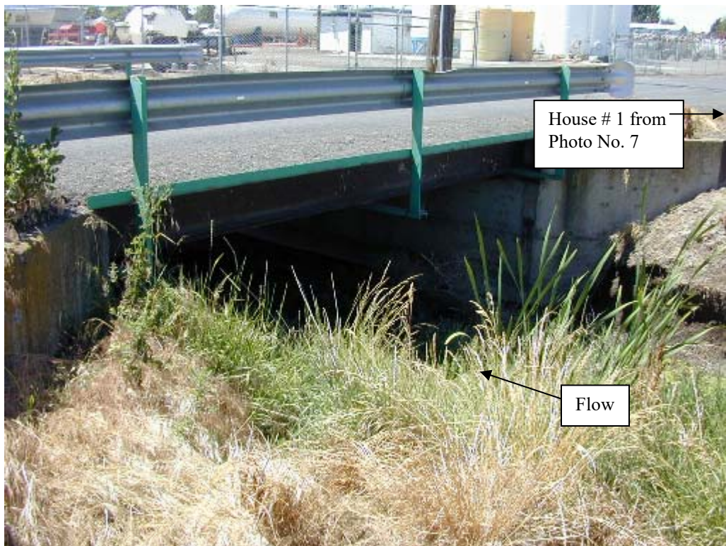
Photo No. 6: View looks downstream at the upstream face of the Sherman St. bridge.
