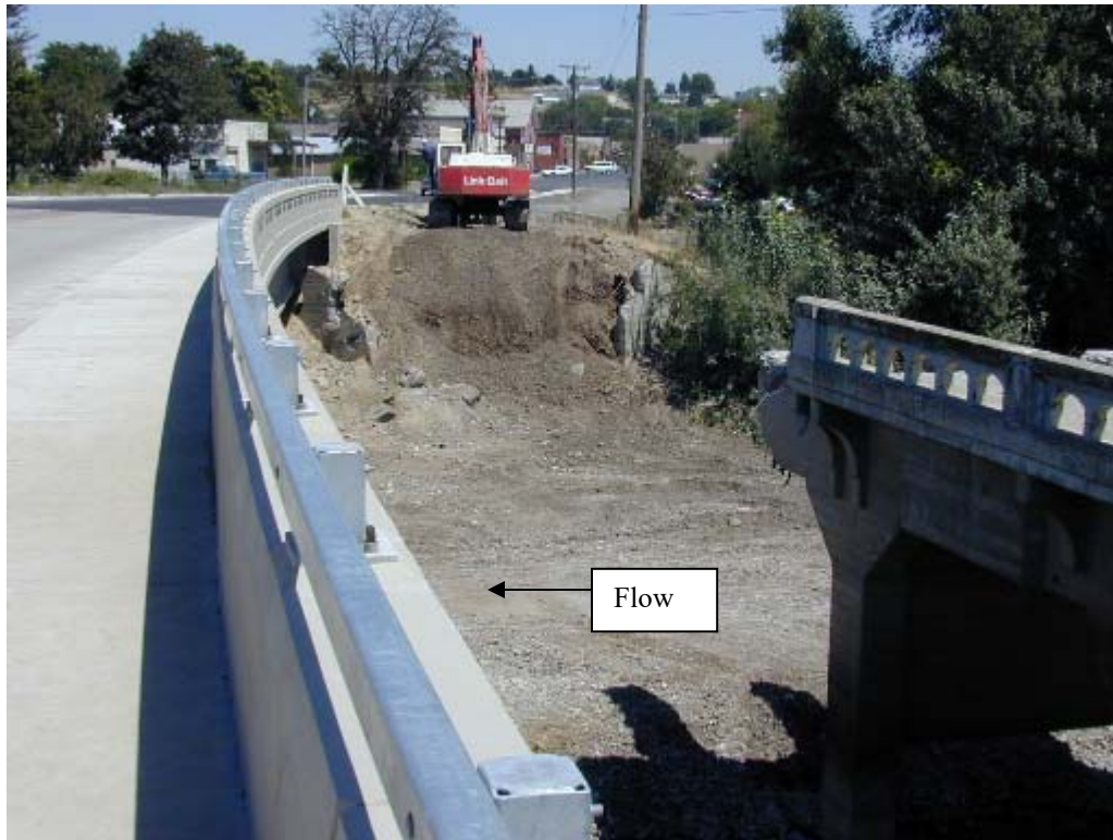
Photo No. 20: View looks north at equipment removing old bridge and downtown area (not in flood plain except lower right corner).
