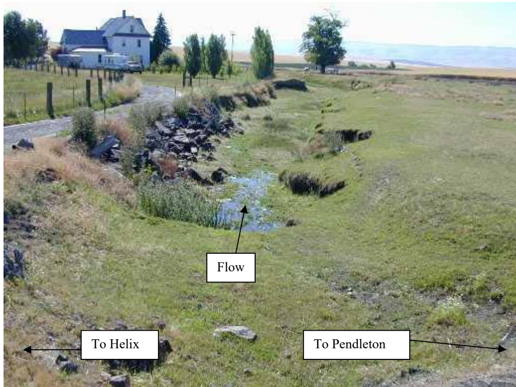
Photo No. 78: View of typical northeastern Umatilla County road crossing. (Actually the Little Greasewood Creek crossing, south of Helix). Looks downstream or southeast.
