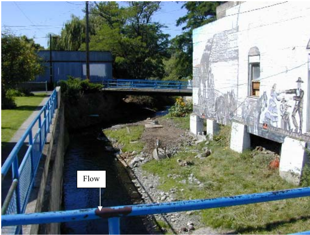
Photo No. 59: View looks upstream (south) at the main stem of Birch Creek from Main St. bridge, showing building encroachment.
