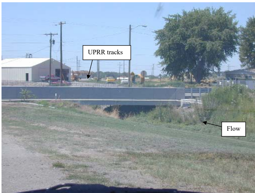
Photo No. 71: View looks downstream (northwest) at upstream face of bridge on SW Sherman St. along west edge of town.
