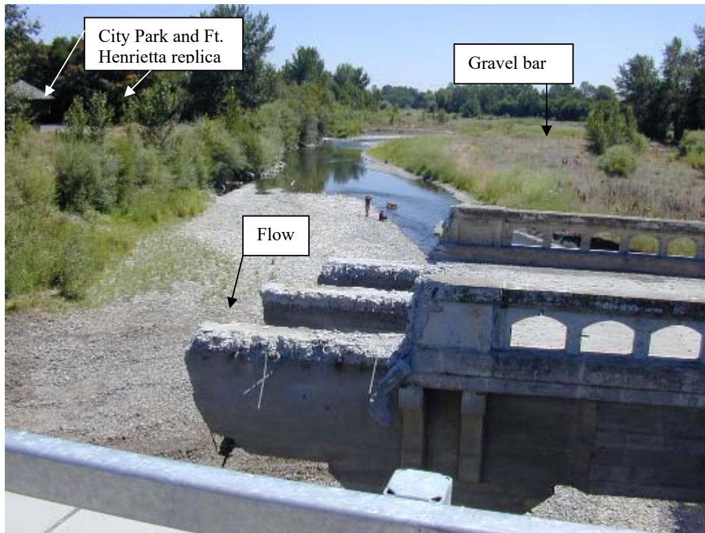
Photo No. 18: View looks upstream (south) at old county road bridge being destroyed and gravel bar buildup west of town. Taken from new bridge.
