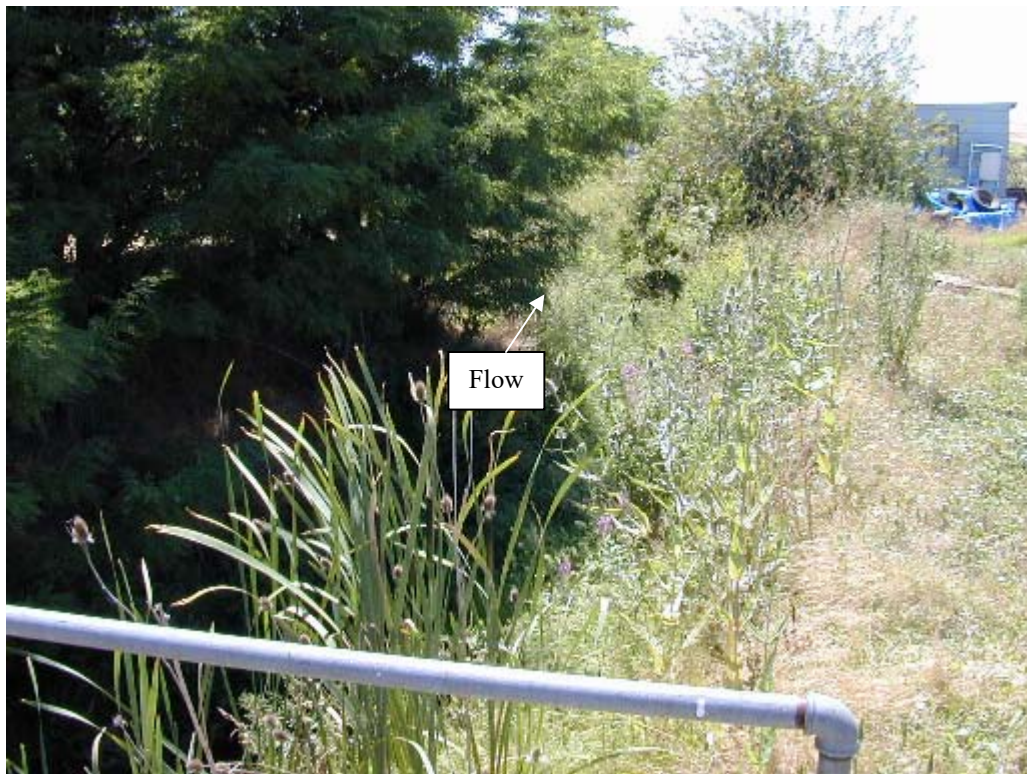
Photo No. 10: View looks downstream (south) at Waterman Creek/Gulch from Main St. bridge/concrete box culvert.
