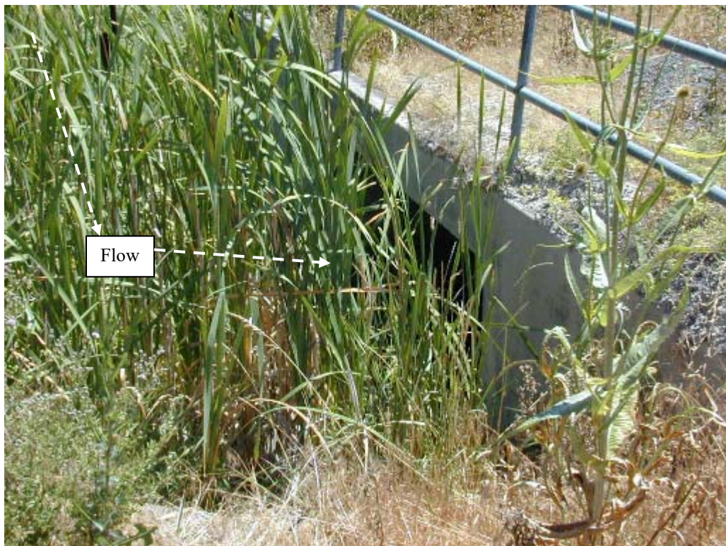
Photo No. 14: View looks southeast at upstream face of Main St. box culvert/bridge.
