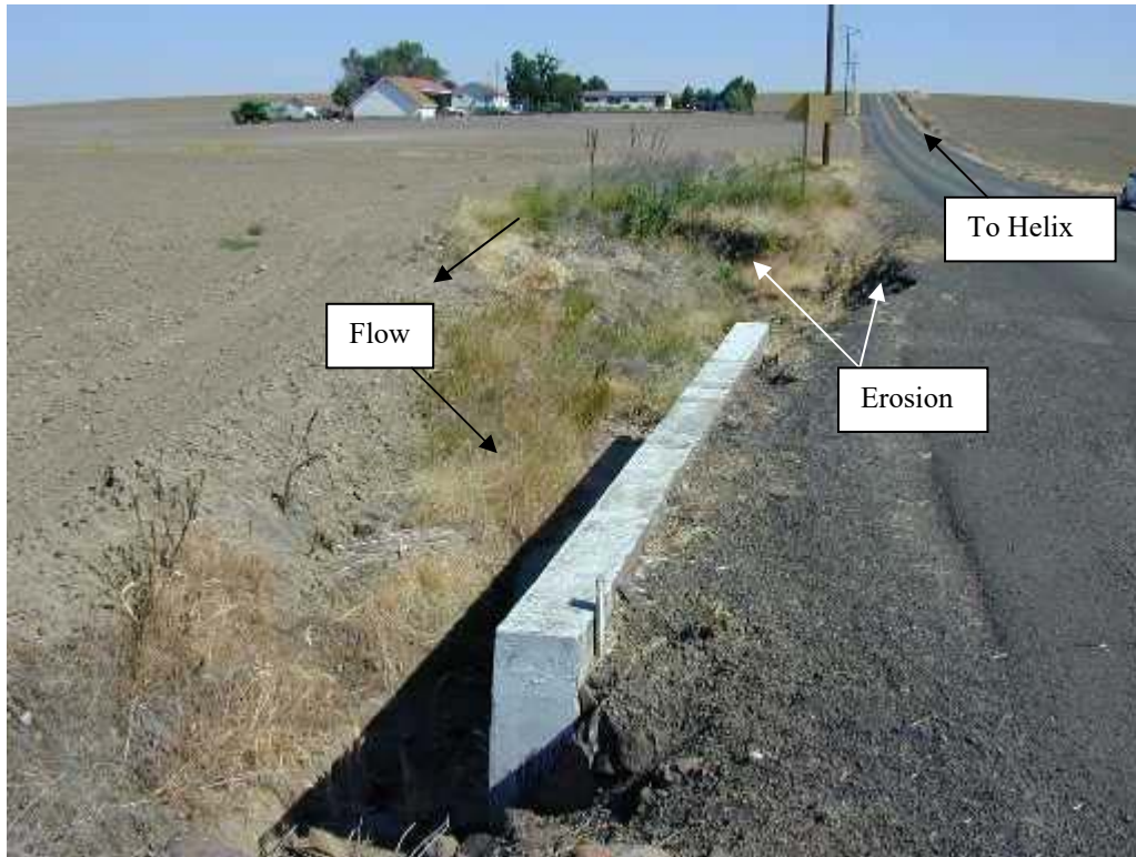
Photo No. 80: View looks at upstream side of culverts showing headwall and county road shoulder erosion caused by high water flow in creek.
